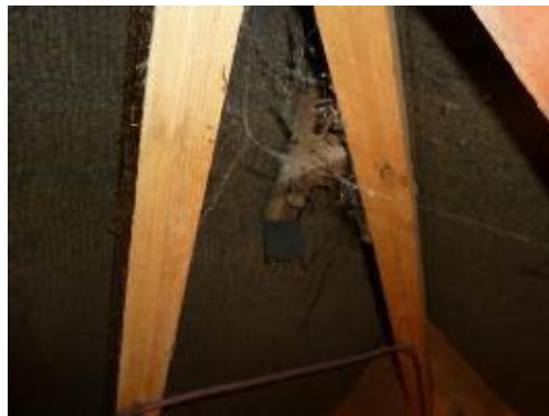
Tear in bituminous lining
